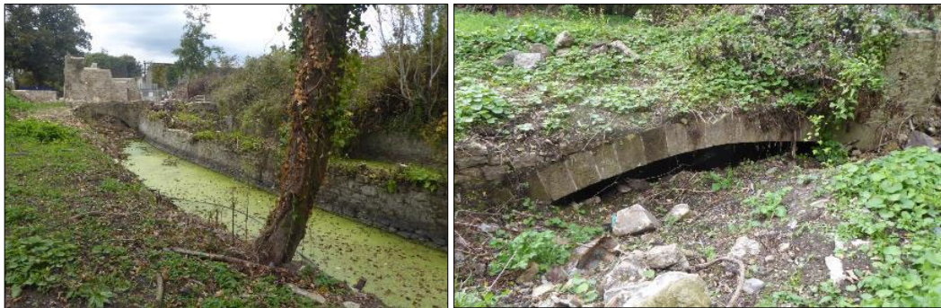
Plate 18 Parallel Tail races view towards west, towards the mill buildings Plate 19 Evidence of a third tail race channel
