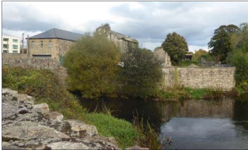
Plate 6 New flood defence walls on the south westernmost end of Suir Island-Willow Island
