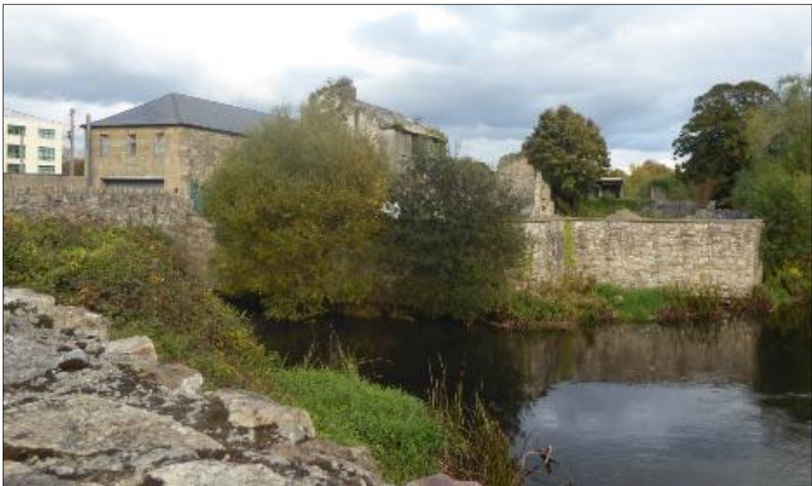
Plate 14-5: New flood defence walls on the south westernmost end of Suir Island-Willow Island
