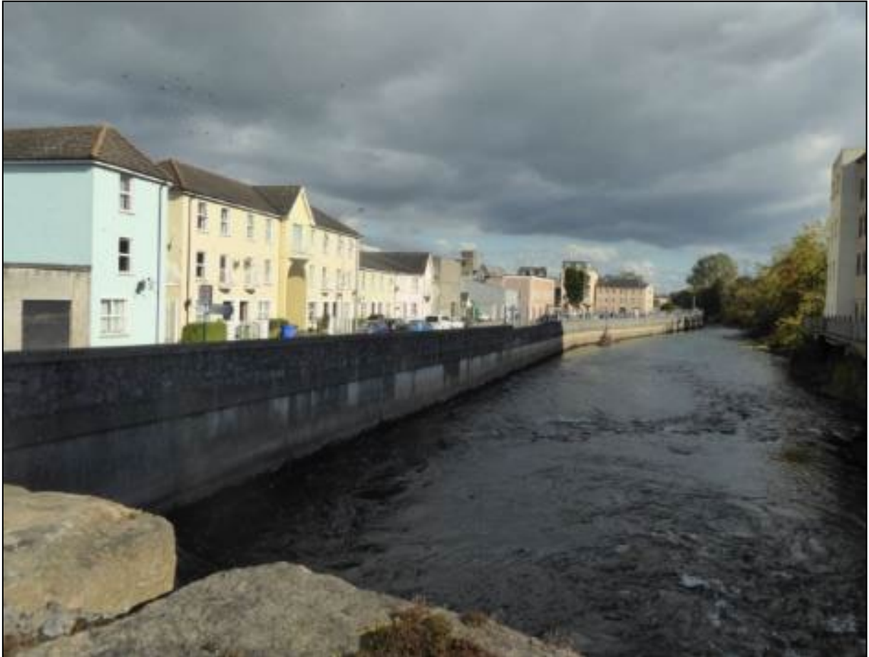
Figure 14-9: New quay walls view form the river from Old Bridge (looking northeast)
