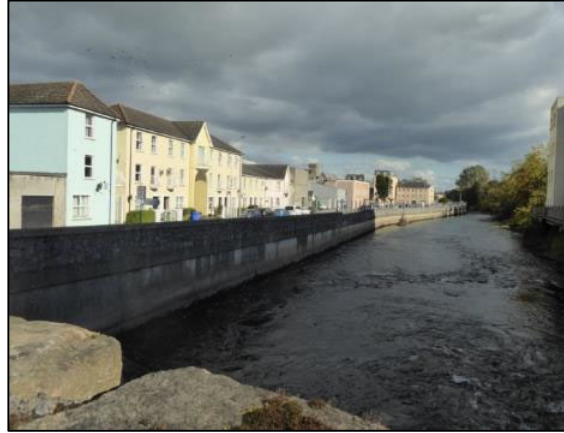
Plate 1 New quay walls view from the river from Old Bridge (looking northeast)
